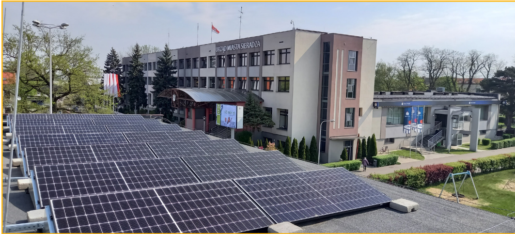
Photo 10. PV installation - Kindergarten no. 1 in Sieradz, 2 Provincial Square Source: Municipality of Sieradz
